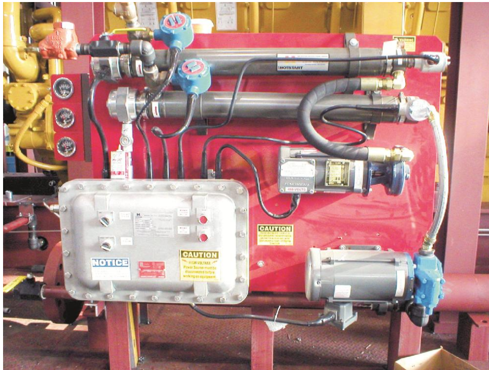
Figure 54: Aftermarket style jacket water heater.
