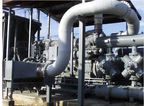
Figure 27: Example of piping with gradual changes in flow direction and self-supporting air intake pipe.
