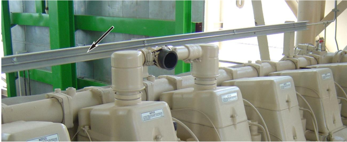
Figure 46: Primary vent line routing. This image shows the cooling system vent line running over the engine. Note the continuous upward slope along the run, and the structural channel used in the installation to protect the tubing from damage.
