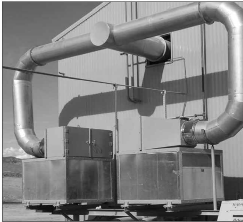
Figure 4.1 – Example of Incorrect Air Inlet Piping Design That Creates Excess Turbulence
