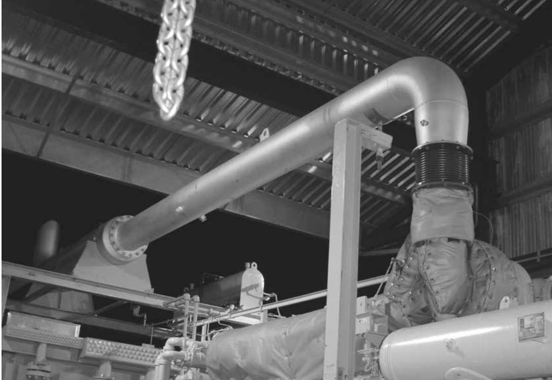
Figure 5.7 – Example of Proper Location of Emission Sample Port in Exhaust Piping
