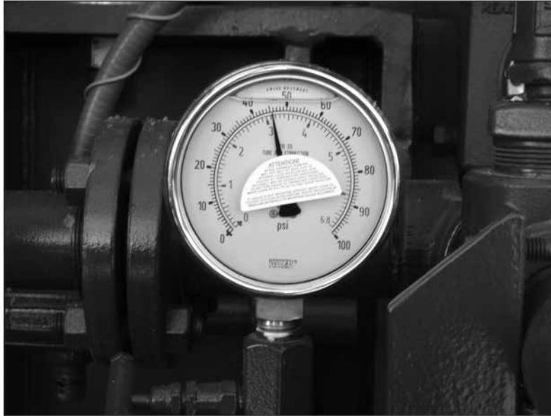
Figure 6.10 – Good Scale Gauge Showing the Correct G3600 Fuel Pressure
