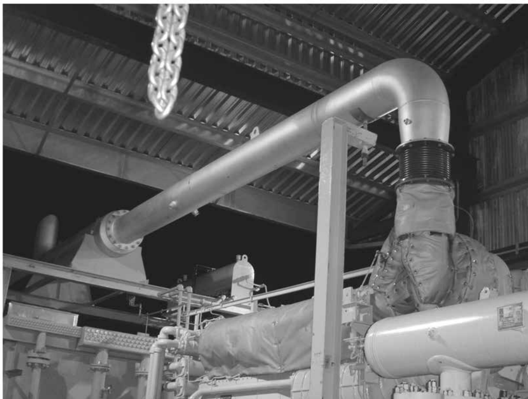
Figure 4.4 – Proper Location of Emission Sample Port in Exhaust Piping
