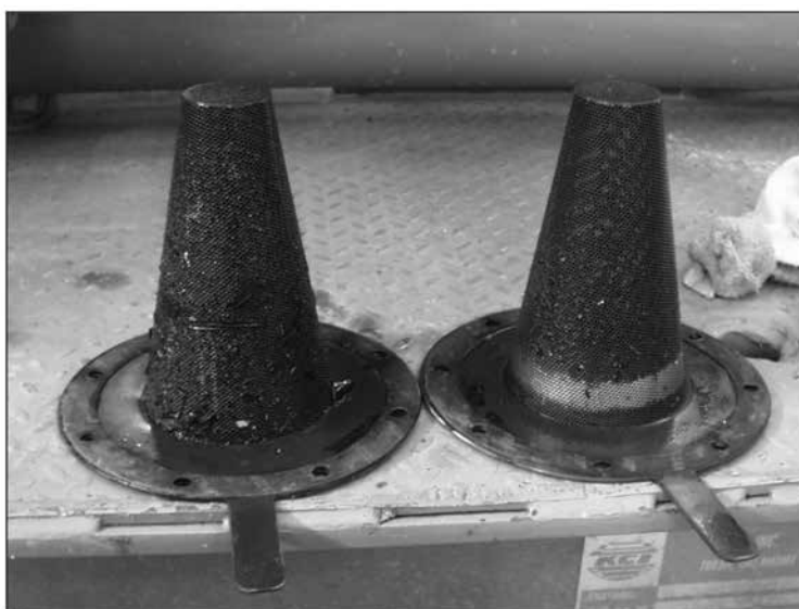
Figure 6.5 – Cat Cooling System Strainers
