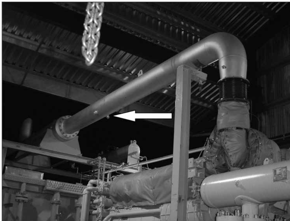
Figure 6.4 – Example of Correctly Located Exhaust Emission Sample Ports
